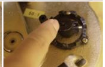
Open status of manual control
